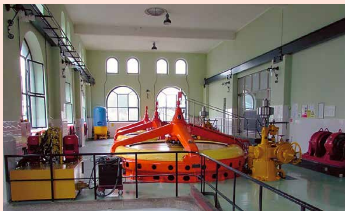
◀ Turbinski agregat u strojarnici HE Ozalj 1 ...
